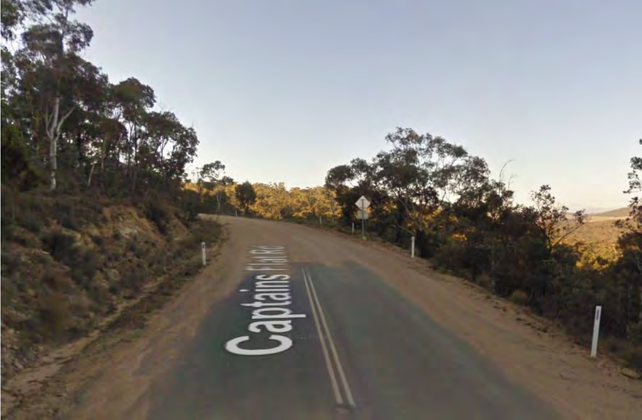
Figure 2: Interface between sealed and unsealed sections of Captains Flat Road located on the southern approach to Captains Flat.
